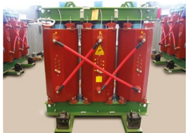
CRT with 7 Regulating points on HV side
